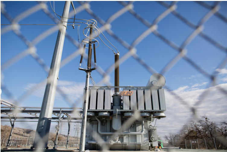
An attack on a PG&E substation near San Jose, Calif., in April knocked out 17 transformers like this one. TALIA HERMAN FOR THE WALL STREET JOURNAL
